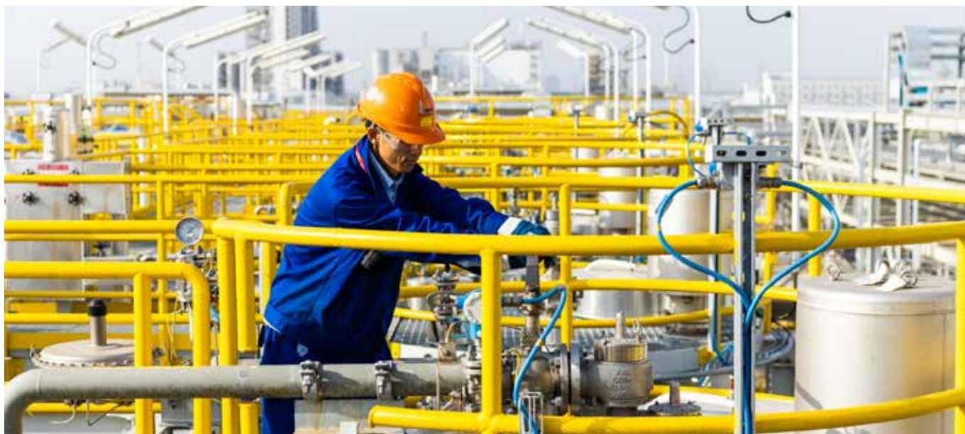
An operator is conducting routine inspection at the Caojing site.
