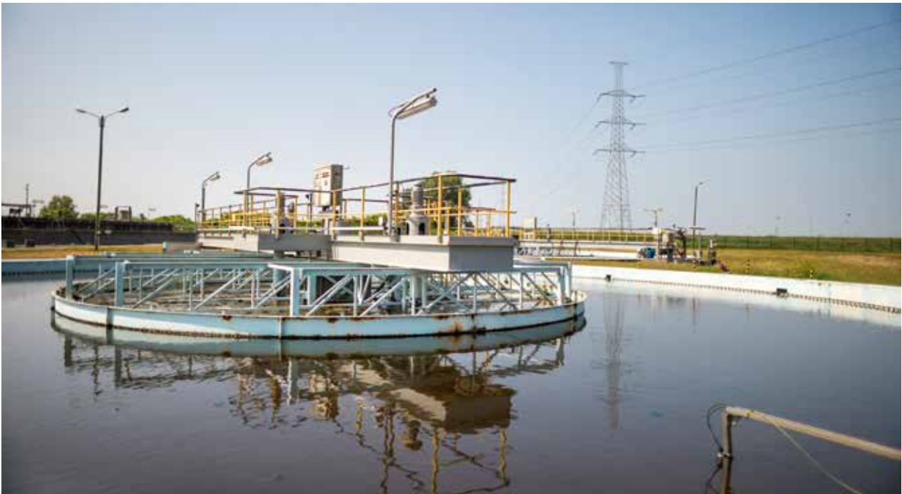
Our water purification plant functions very well.
