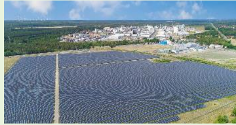
On-site solar park Schwarzheide, Germany
