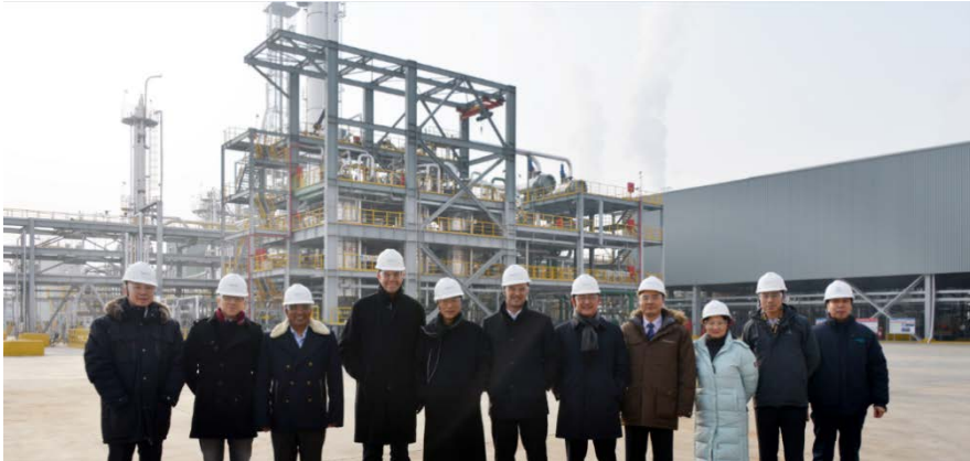
Start-up of butanediol plant at the integrated PolyTHF complex in Korla, China
