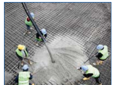
Glenium® makes concrete more flowable: contractors can pour the foundation slab in record time. Photo: Klaus Helbig
