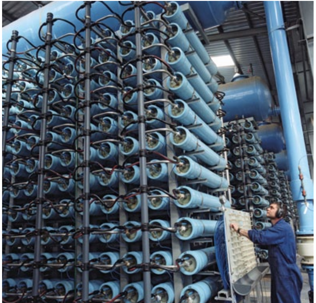
Right Desalinated seawater from plants like this one in Cyprus could be providing water for 14% of the world's population in 2025, according to industry experts.
